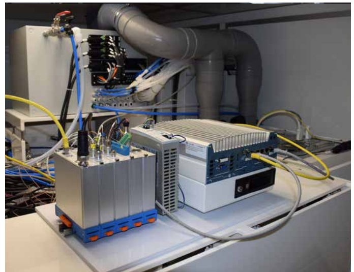
The KiDAQ data acquisition system from Kistler (front left) is connected to an IPC (front right) that initially provides temporary local storage for data from the plant.
